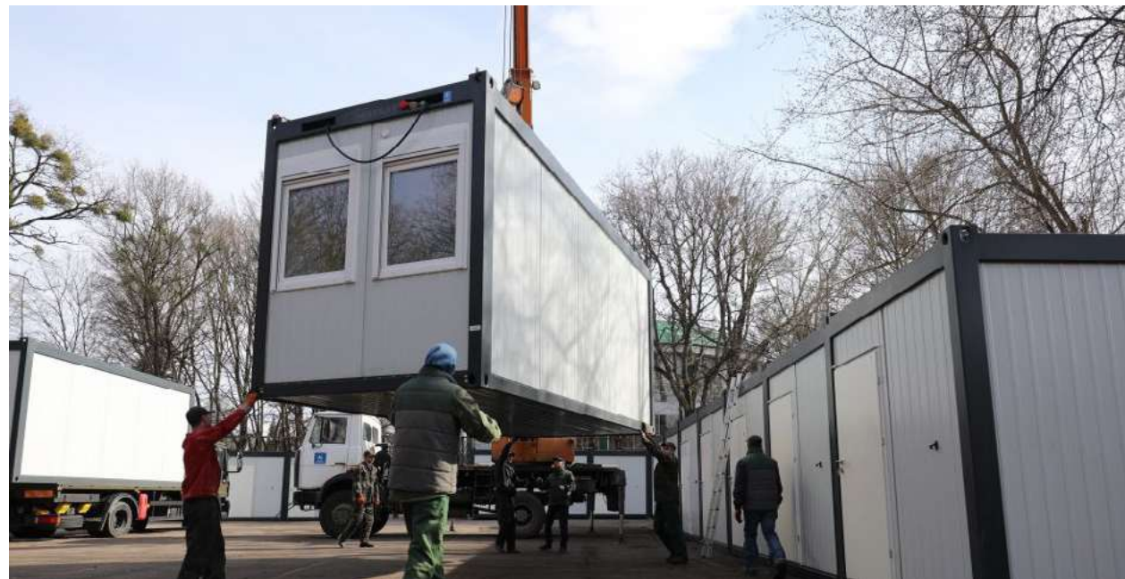
[Fig. 54] Case Study a05 Residential Camp 1 made with shipping containers © Roman Baluk
