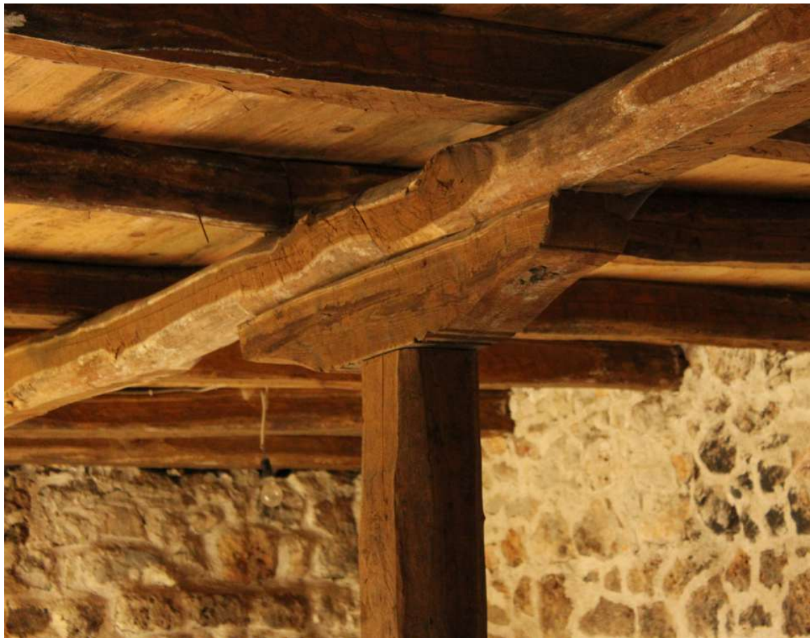
Fig. 144 The wooden construction of the first floor, Mill of Ali Bel Bicaĵ
