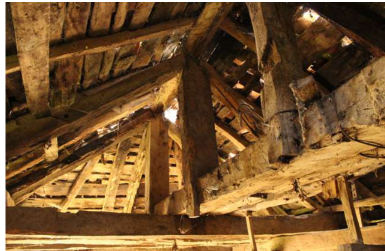
Fig. 92 (left) Close-up image of the wooden roof construction at Mill in Glllogovica, Glllogovica, Prishtina
