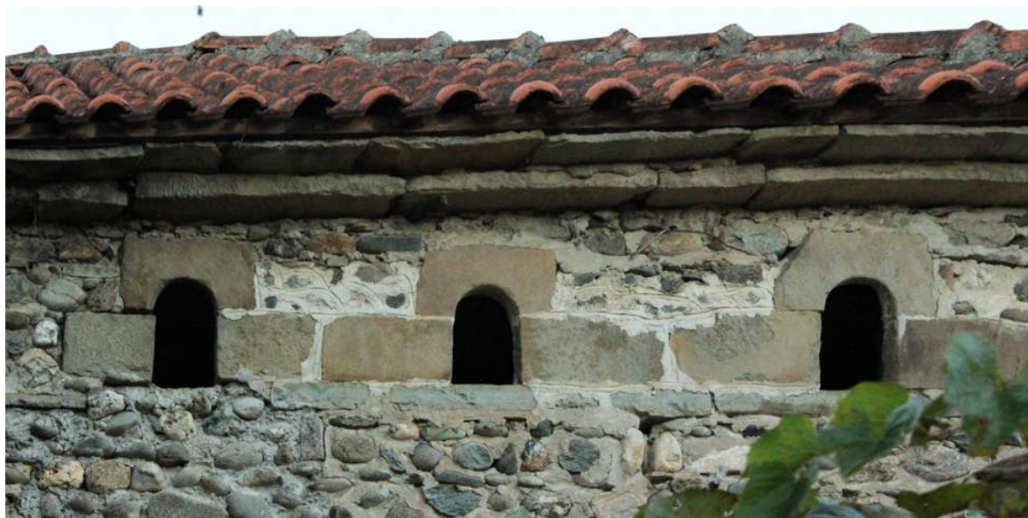
Fig. 125 Close-up image of the second floor windows on the rear facade at the Mill of Sylëregja family
