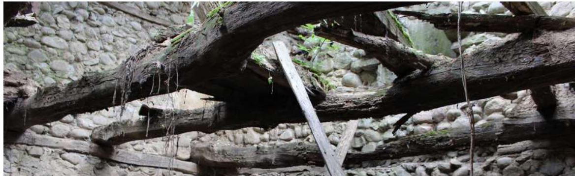
Fig. 233 View from the almost destroyed structure inside the mill of Mill of Mehmet Bricori, Kamenica, Peja
