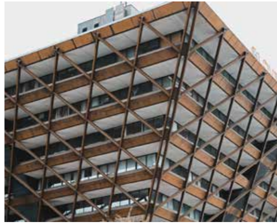
Fig.2 Slovak Broadcasting Building, Bratislava Slovenský Rozhlas Štefan Svetko, Štefan Ďurkovič, Barnabáš Kissling 1962 - 1985
