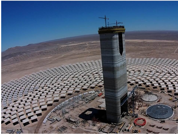
Figure 1.1.: Picture of the construction side of the 110 MW Cerro Dominador CSP plant in Chile with storage tank basement in 2019 [121]
